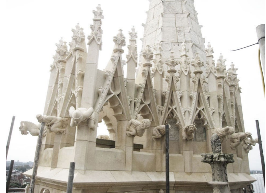
Figure 29 - An example of completed stonework after conservation works carried out by stonemasons, Andrew Arrol
