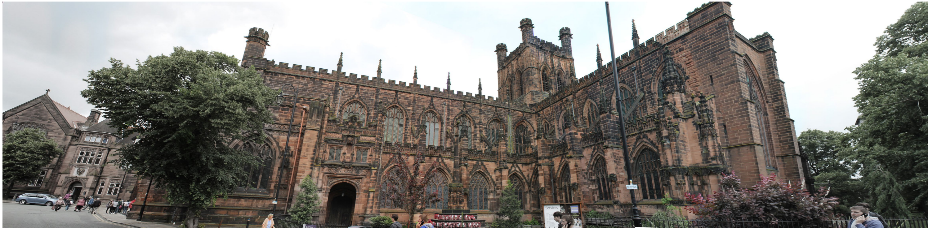
Figure 48 - External view of Chester Cathedral indicating various levels of weathered red sandstone, Author's own
