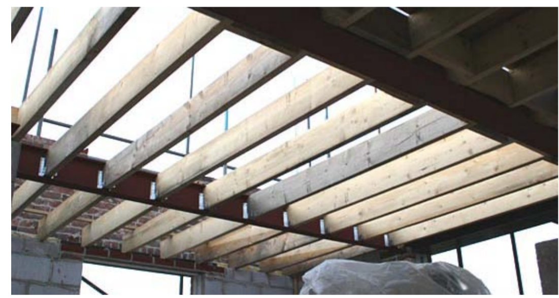
An example of a building under construction with timber ceiling joists in place
